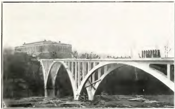
Construction view showing incomplected footbridge being built by us for Washington and Lee University. This bridge connects the campus with the athletic field.
