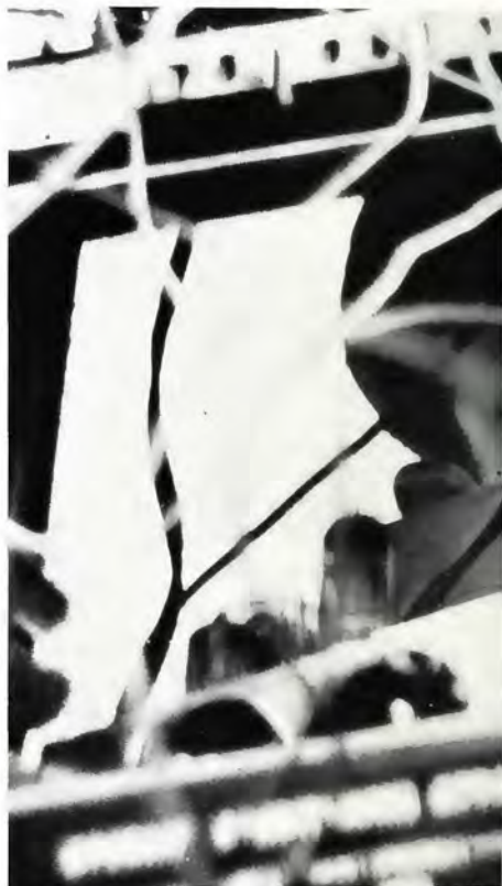
Wiring maze presents complex problems.
