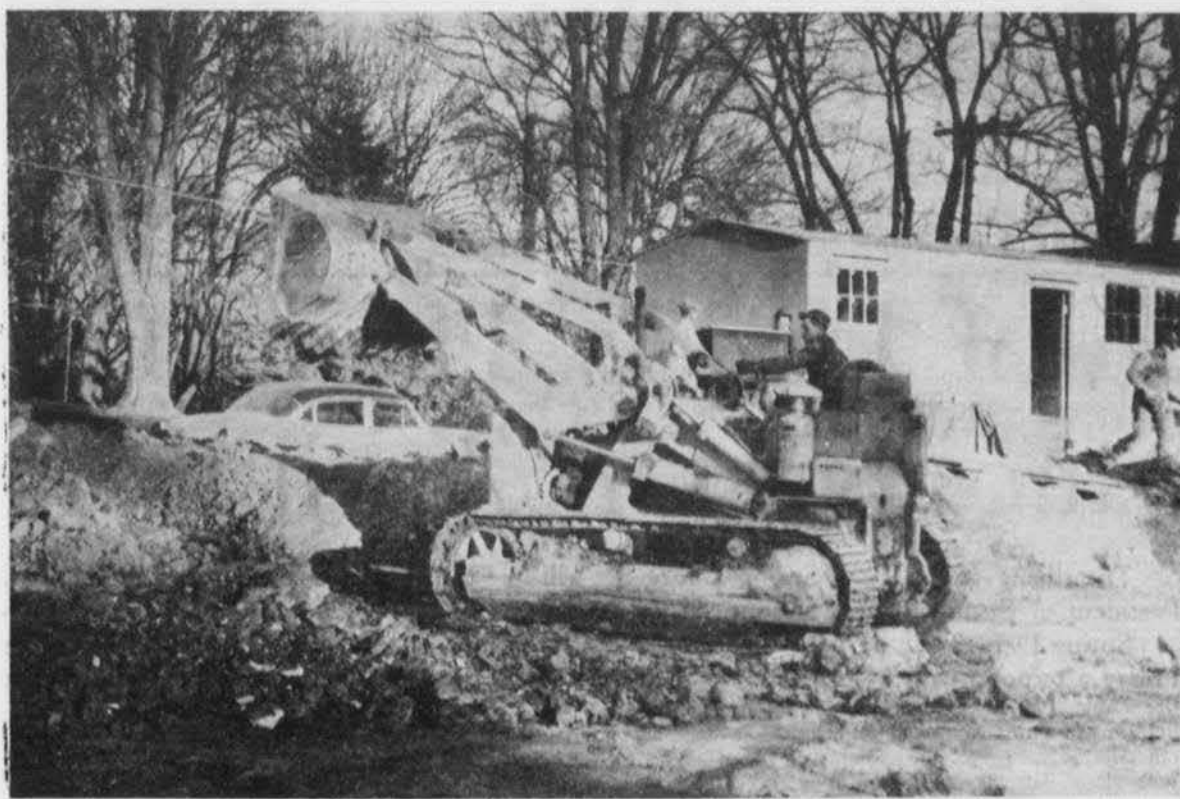
PROGRESS CONTINUES in the construction of the University Commons-Dorm despite foul weather. Each additional step in the construction of the new structure diminishes the time to make fraternity adjustments.
