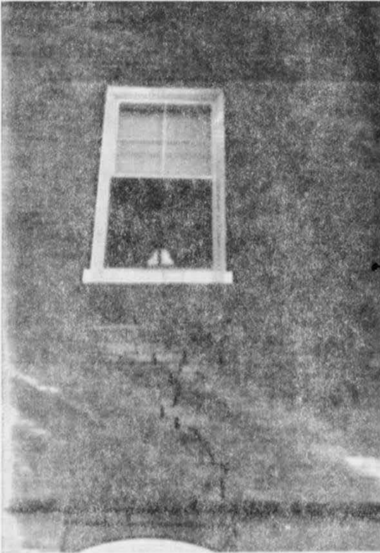
The fissure on the east side of the Commerce School continues to widen, indicating the structural weakness of the building. The crack will go unrepaired until funds are available for refurbishing the structure.
