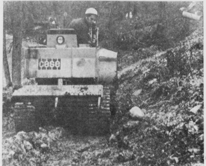
A construction worker levels out the hillside near Woods Creek as part of site preparation for the student apartment complex to be completed by this fall.
