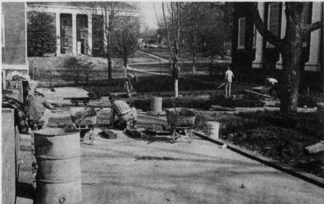
This week's warm weather has helped speed the landscaping work on the back-campus. photo by Chris Volk
