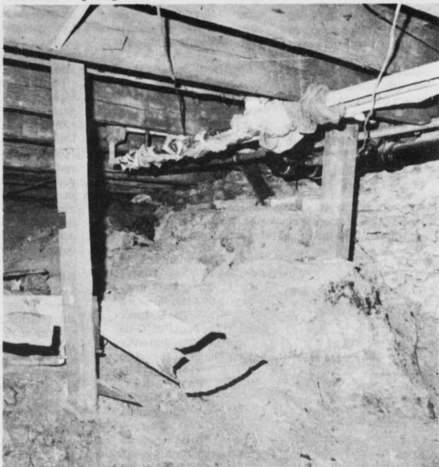
Makeshift insulation protects these waterpipes from freezing winter temperatures, but a plumber has said that the insulation is inadequate.
