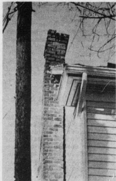
A builder has said that this chimney will fall.
