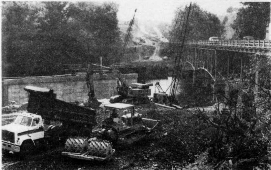
Bridge building —Work is in full swing on a new bridge over the Maury River just outside Buena Vista on Rt. 60. (Staff photo by Kevin Berger.)
