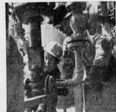
MAINTENANCE TEAM making a speedy change of a methanol valve to minimize production loss.
