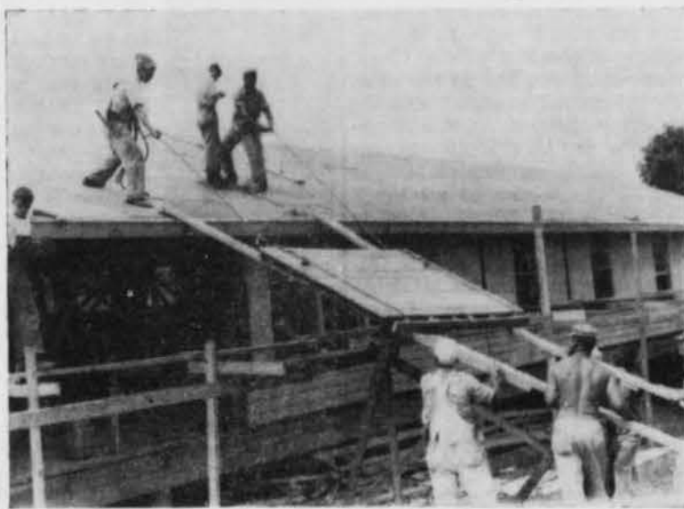
Construction was moving according to schedule at Davidson Park student housing project last week. Workmen are shown above hoisting a pre-fabricated roof section into place on a five-unit house. Staff Photo by Phillips
