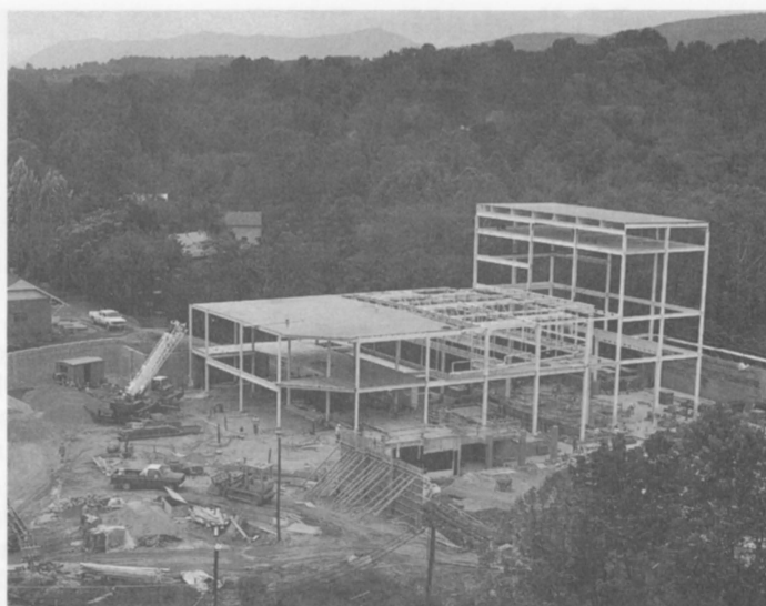
Construction on the Lenfest Center for the Performing Arts is proceeding on schedule and is expected to be completed by September 1990. The center will be named for Marguerite and Gerry Lenfest, '53, whose gift of $3 million is helping to finance the project.
