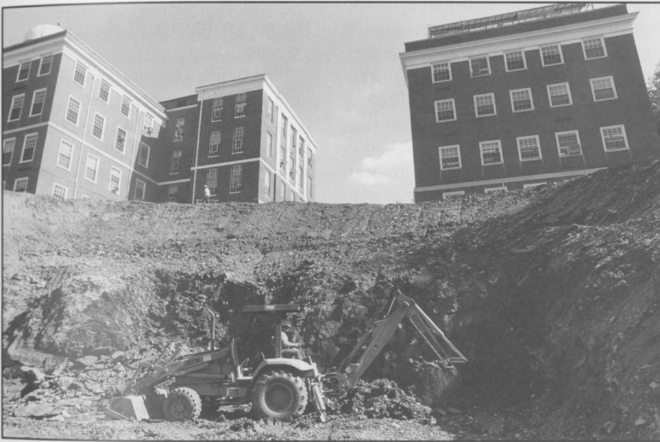
Digging deeper: Construction is underway for the new science center, which will link Howell (left) and Parmly halls. The project, ticketed at $21 million, will be paid for by gifts to the capital campaign.
