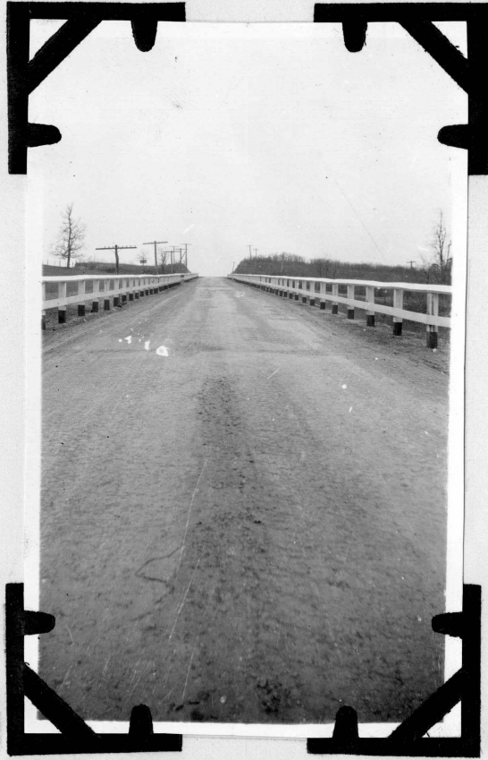
Rough suriace due to bad grading.
