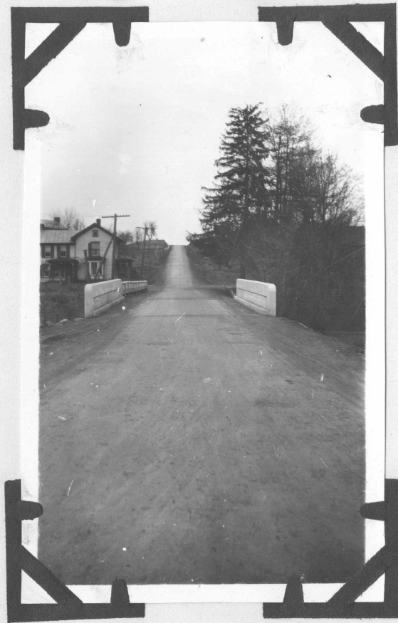
Settlement of fill at either end of bridge due to not tamping.
