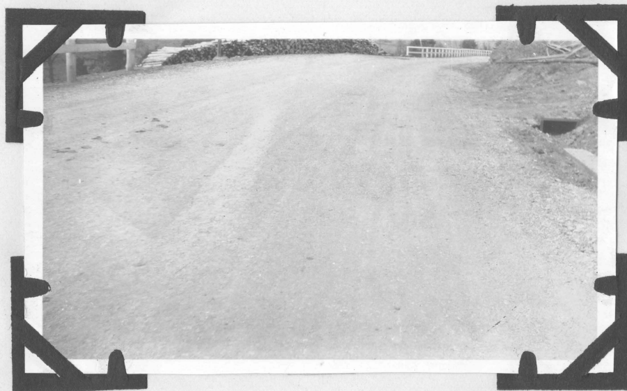
Hole in macadam due to bad seal coat.
