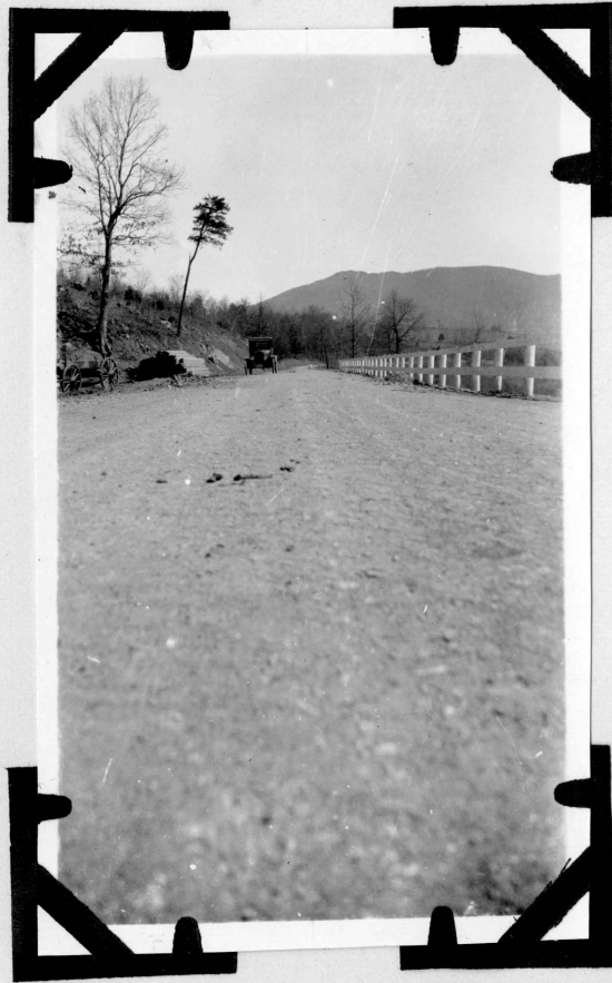
Settlement of surface due to rill settling.
