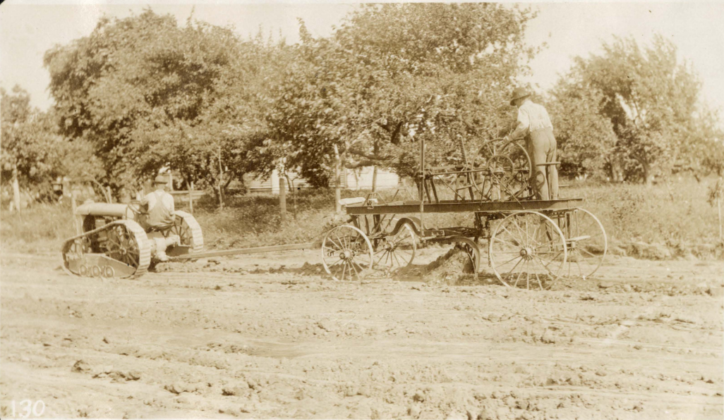
SMOOTHING UP MATERIAL THAT HAS BEEN PULLED LOOSE BY LARGE TRACTOR OUTFITS.
