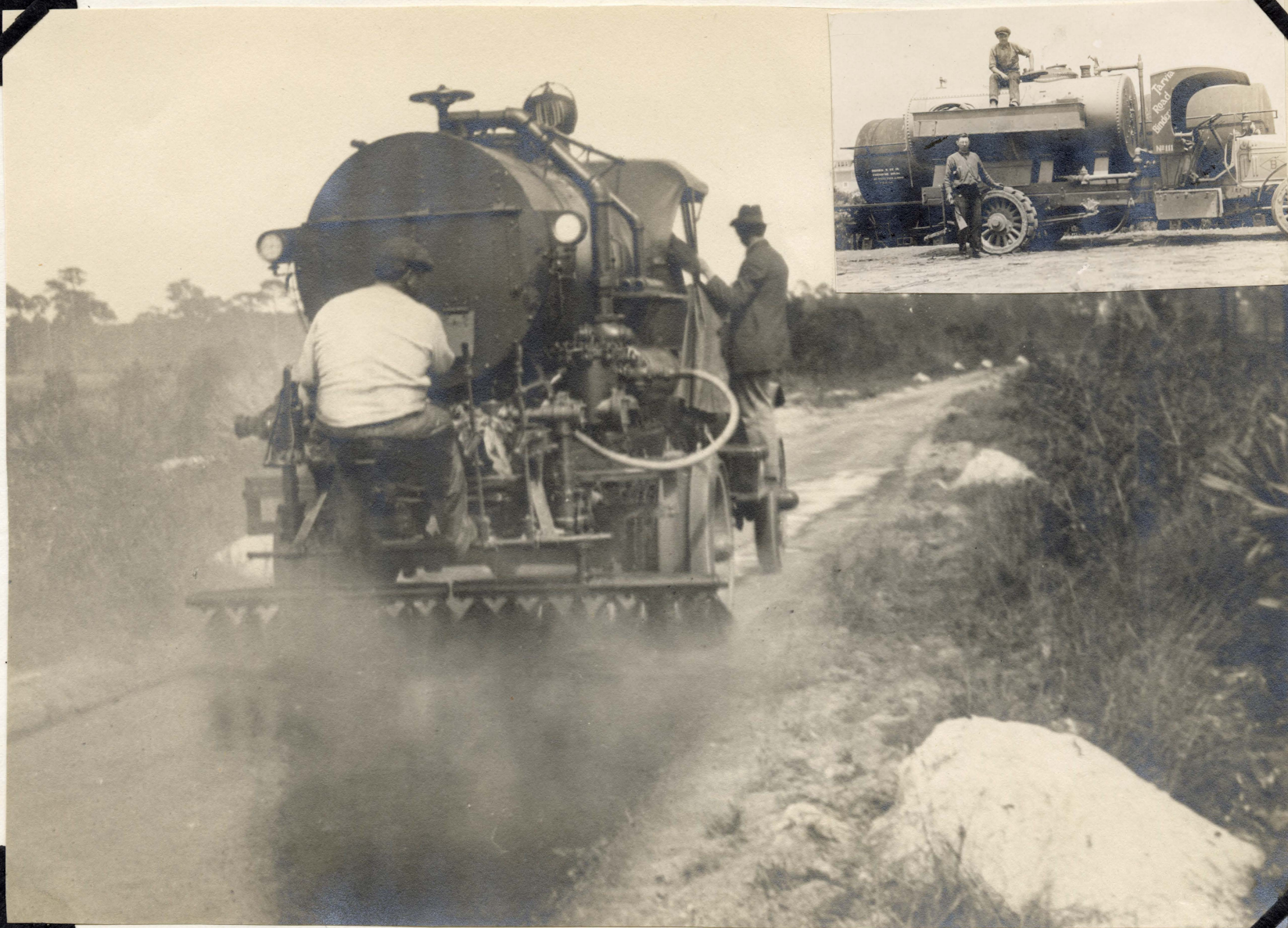
MOTOR DISTRIBUTOR MAKING APPLICATION OF BITUMINOUS MATERIAL ON MACADAM ROAD. (Insert) LOADING DISTRIBUTOR FROM TANK CAR
