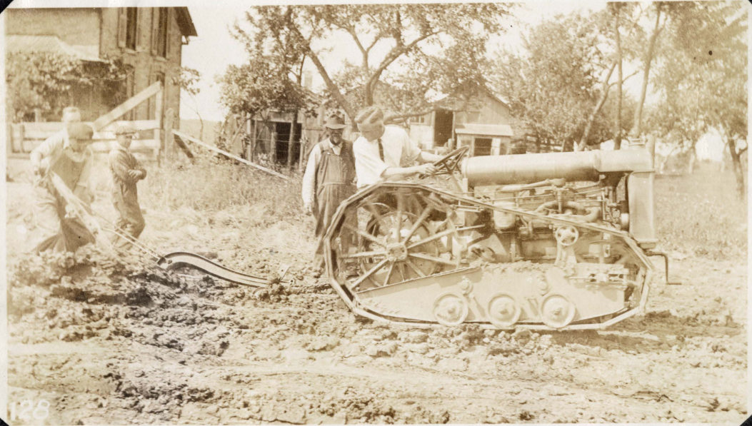
USING TURN PLOW TO BRING UP NEW MATERIAL INTO THE SURFACE OF A SAND-CLAY ROAD.
